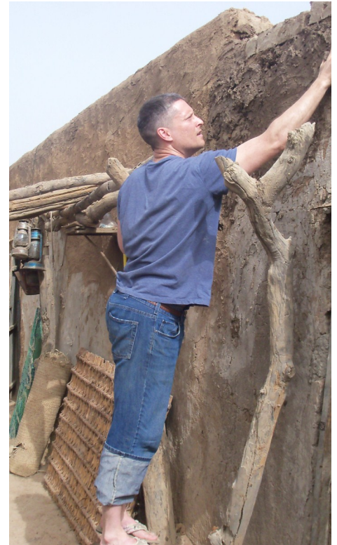
Steve Hilton working on a mud hut in Mali. How do you repair a mud hut? With mud!!!
